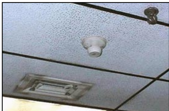
Smoke detectors should be at least three feet from HVAC diffusers
