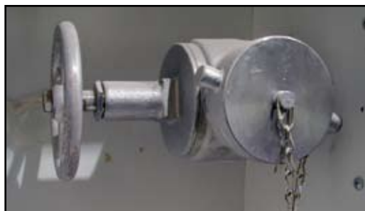
Typical Class I hose station outlet.
