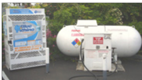
This LPG cylinder exchange rack should be at least 20 feet (6096 mm) from the dispensing equipment.
