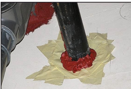
This wall penetration should be sealed in accordance with manufacturer's recommendations. Photo courtesy Sam McLain, Johnson City, TN.
