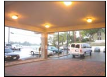
There is no fire sprinkler protection in this drive-through porte-cochere.
