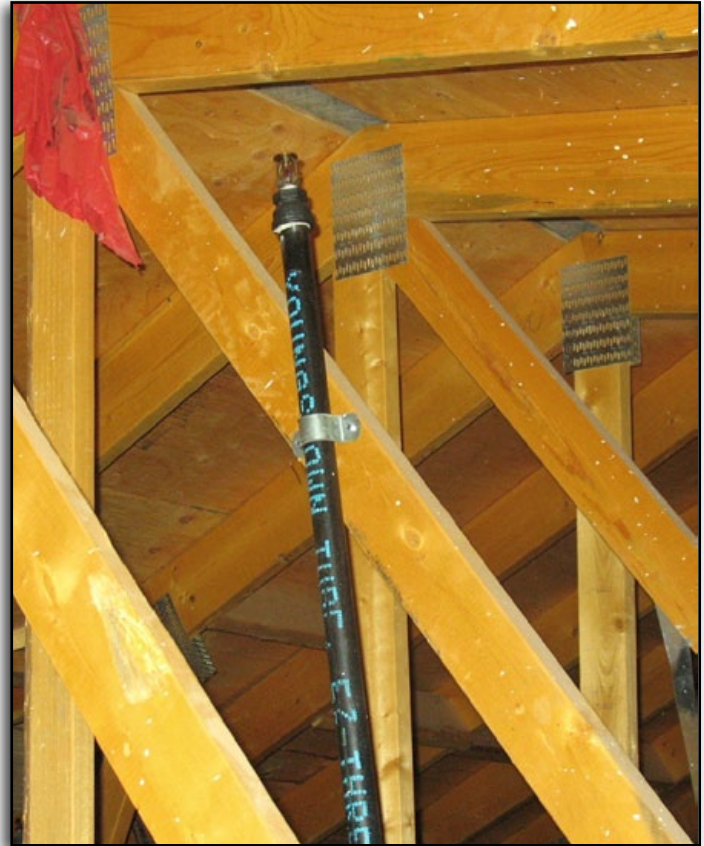
Photo courtesy of Freedom Fire Protection, LLC, Longmont, Colorado. Because of its length, this sprig must be supported to restrain lateral movement.
