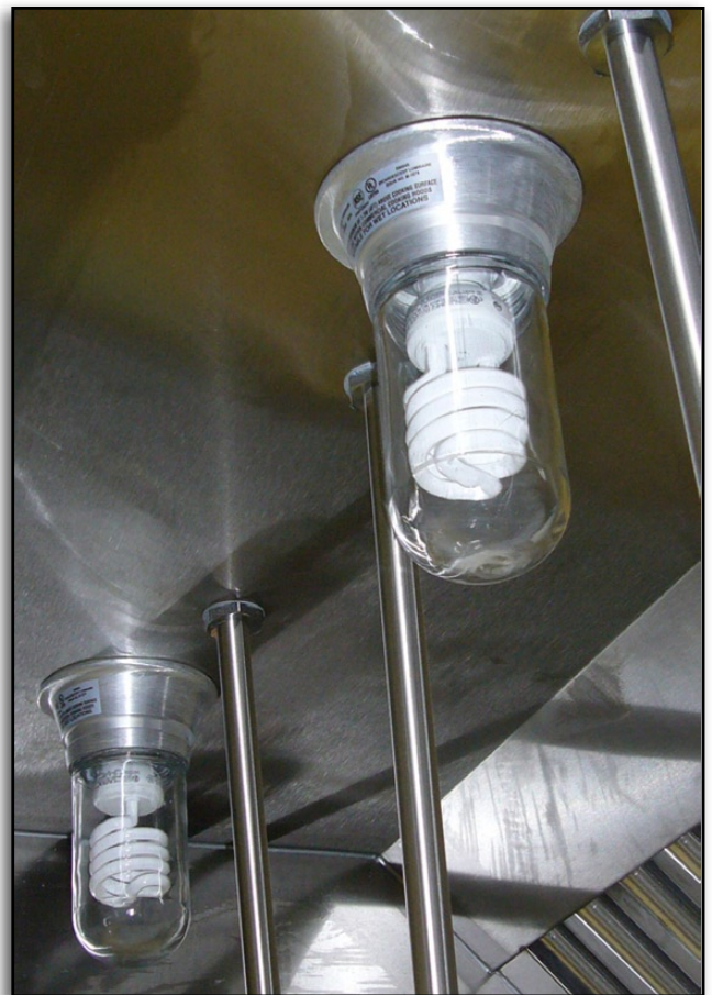
These in-hood luminaires must meet strict guidelines to prevent a fire.
