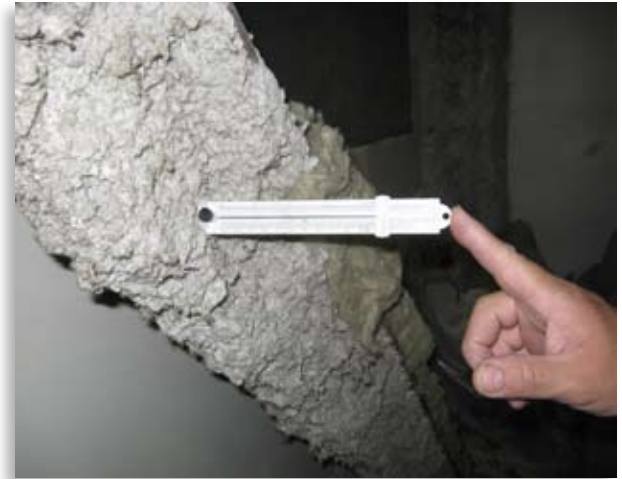
A special inspector checks the thickness of spray-on fire-resistant materials on a structural element.
