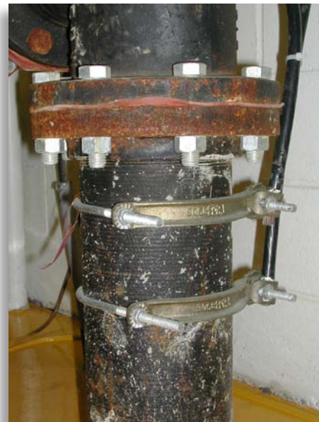
This sprinkler riser is appropriately bonded to the metal building in which it is located.
