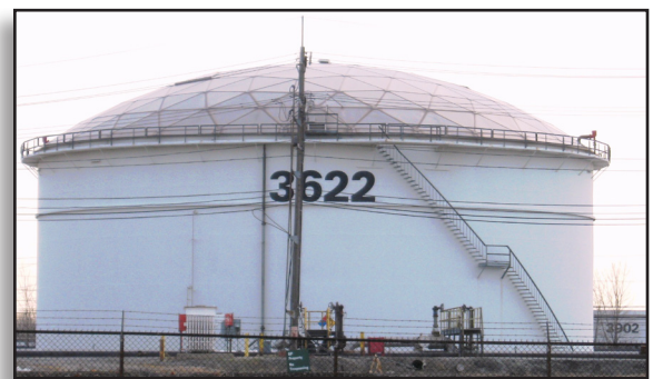
This bulk petroleum tank geodesic dome roof is made from noncombustible aluminum.
